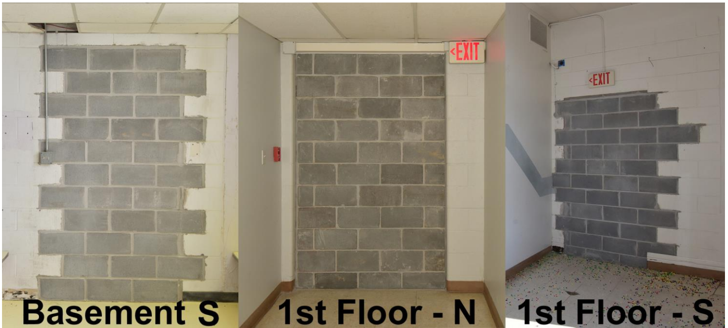
Figure 23. Infilled former entrances to the 1981 pool addition. Left image is from the south entrance in the basement; center image is from the first-floor north entrance; the right image is of the first-floor south entrance. Source: Brad Finch, f-stop Photography, December 2018.
