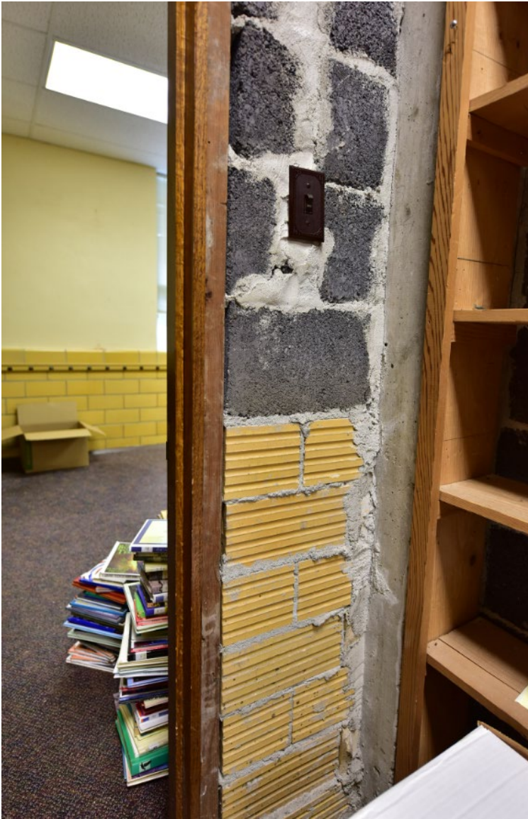
Figure 8. Detail of wall construction, showing structural clay tile below and Cinder Blox (name brand) above; plaster applied to the cinder blocks on the room-side of the wall. Source: Brad Finch, June 2021.
