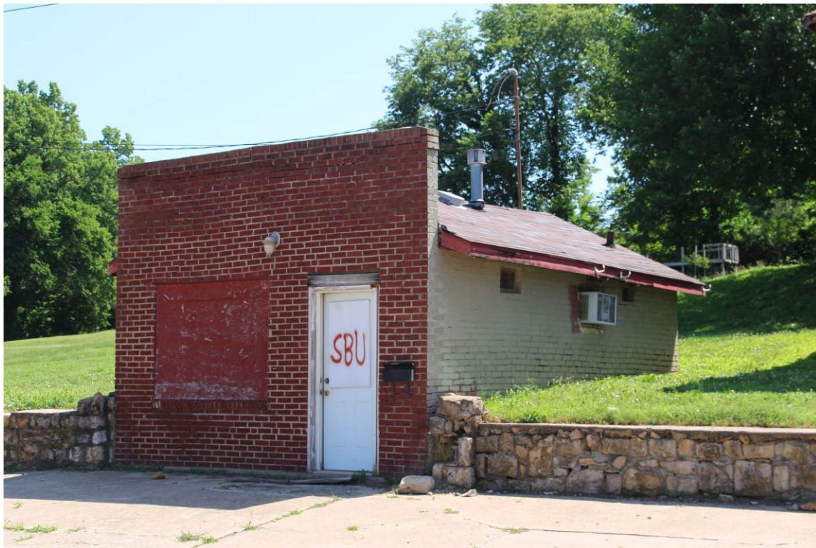
Figure 3 Garage, West (main) and south elevations. View of the stone retaining wall.
