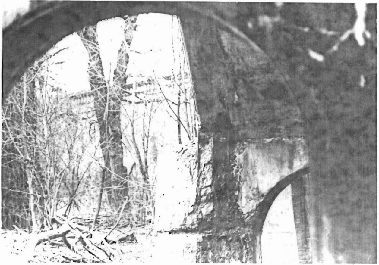
Cottonwood River Bridge detail of pier damage.
