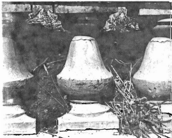
Cottonwood River Bridge blacktop oozing through railing.
