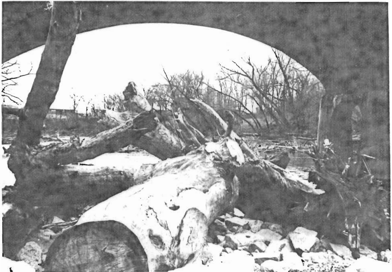
Cottonwood River Bridge drift collecting underneath span.
