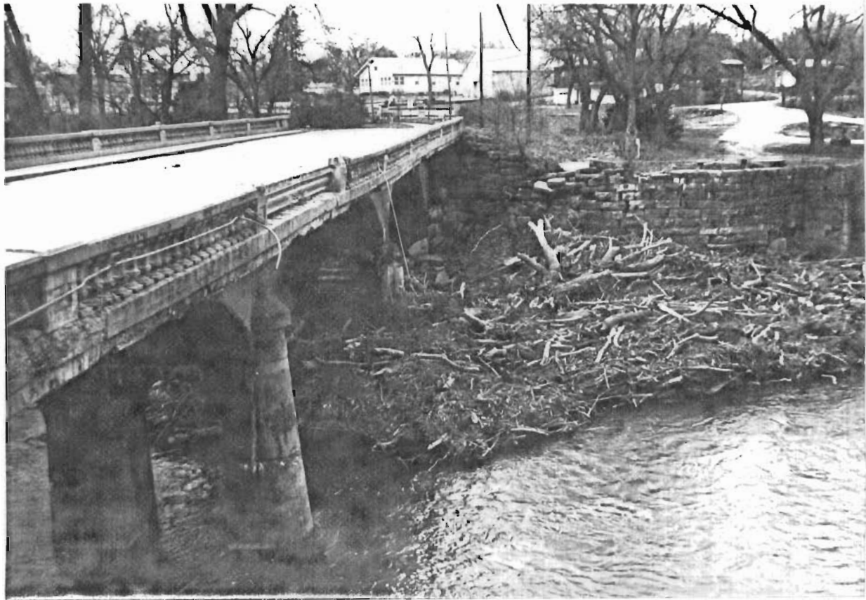
Cottonwood River Bridge west side looking south showing backed up driftwood.
