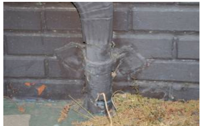
Some of the original downspout straps remain
