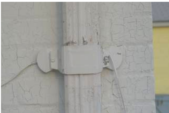
Downspout strap on garage addition
