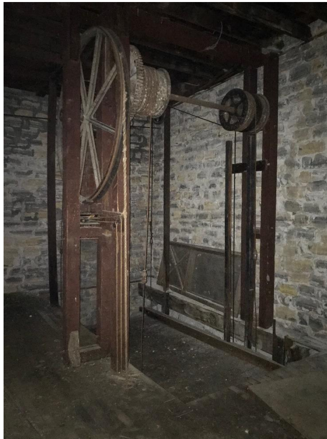
Photo 31: Elevator mechanism for 149 Wabash
