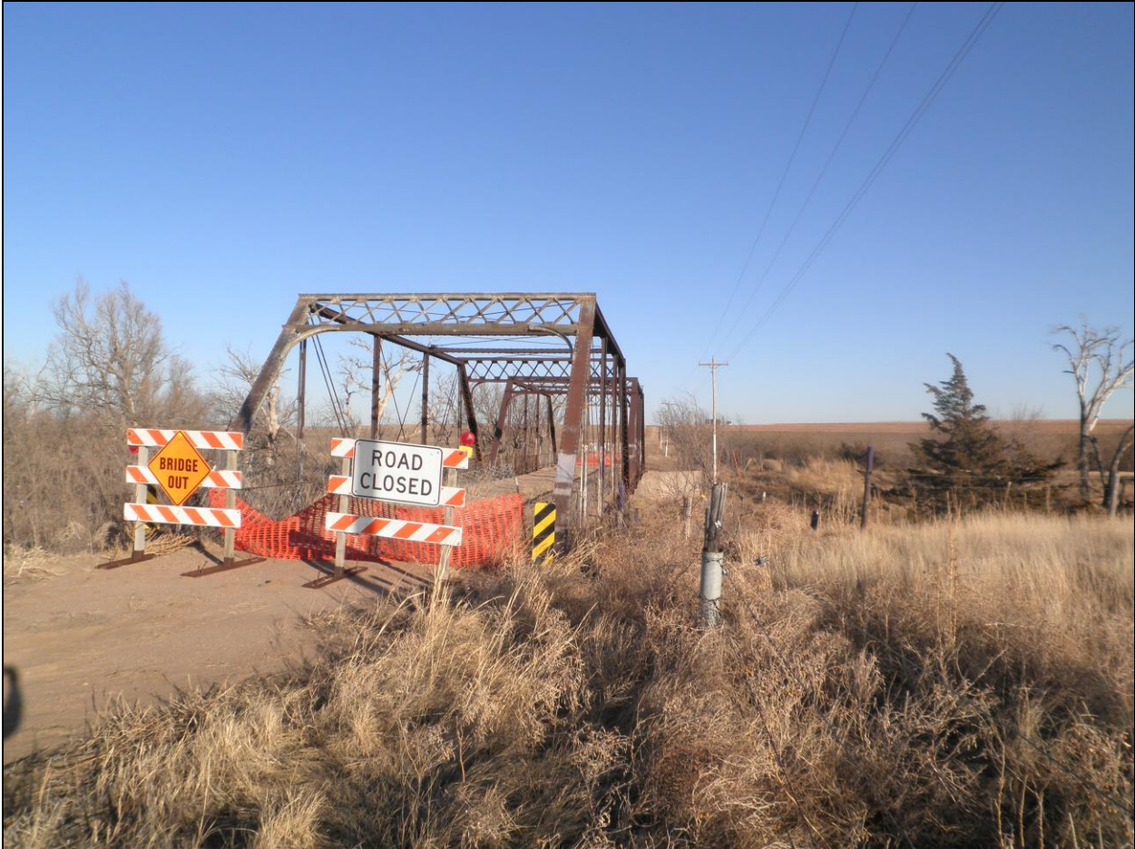
Figure 3. Mulberry Creek Truss Bridge looking east-northeast. Photograph taken on January 21, 2014.
