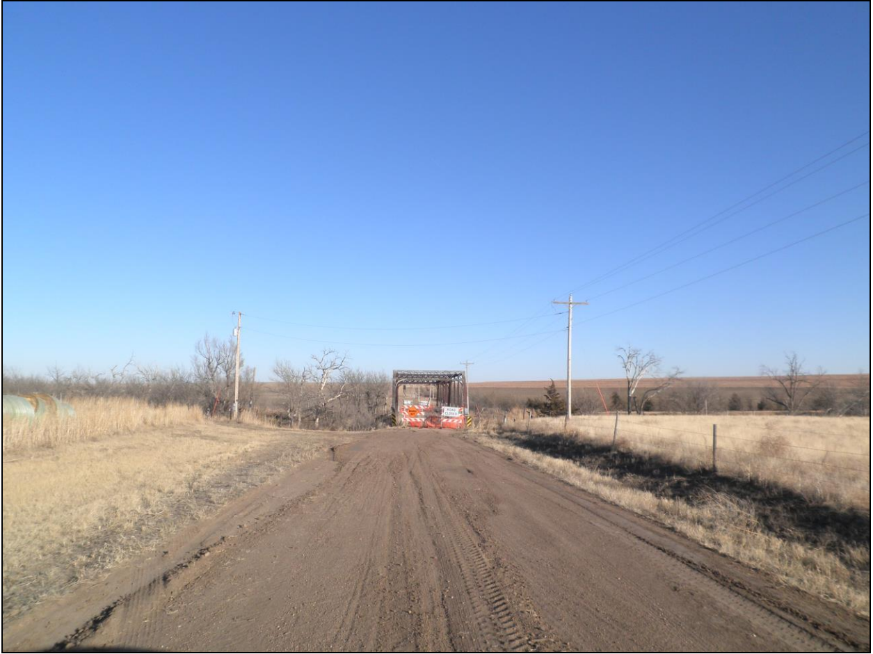
Figure 1. Overview of Mulberry Creek Truss Bridge looking east. Photograph taken on January 21, 2014.
