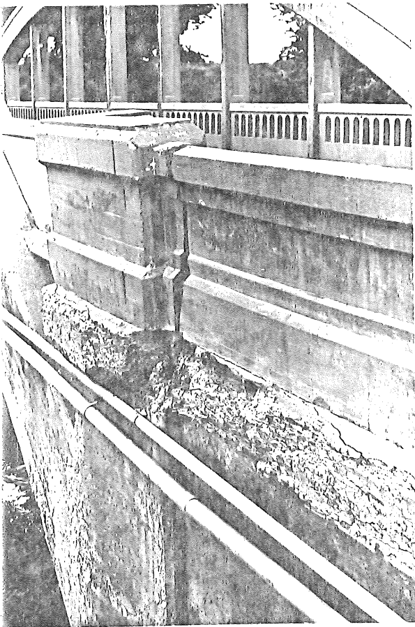
Cottonwood River Bridge North side of the west end showing spalling of concrete.
