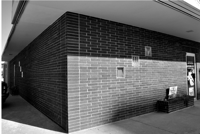
FIGURE 20: Current view of 113 North Norton Avenue. Detail of uncommon embedded glass block elements
