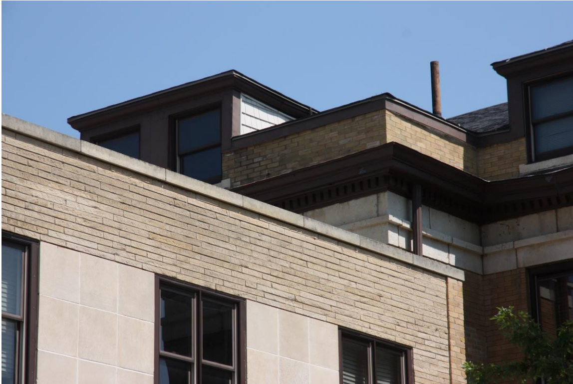
Close-up of stone (or concrete) work at upper story of south elevation of 1958 addition, looking up from the southwest.
