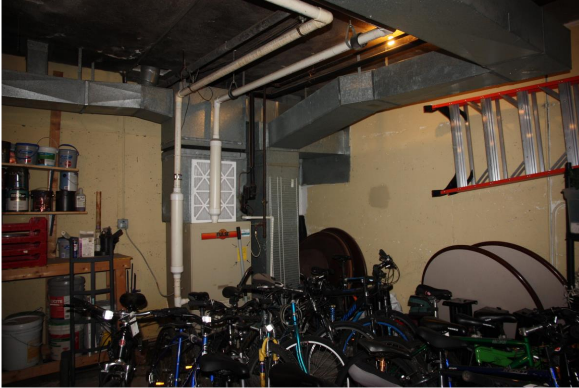
Basement Mechanical Room, looking southwest.
