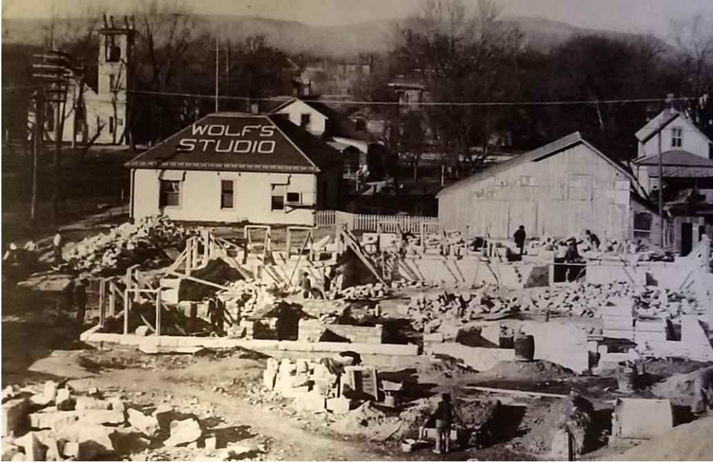
Figure 7 - RCHSM Photo, ca. 1905, View of Wolf Studio with roof sign from east during construction of courthouse
