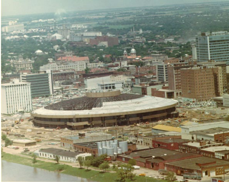
Figure 23 - Century II under Construction with R.H. Garvey Building in background on left Unknown photographer, 1968. Archives of the Wichita Area Chamber of Commerce, Wichita State University Libraries, Special Collections and University Archives . Digitized 2003 (wsu_ms2002-12.68.54.4).
