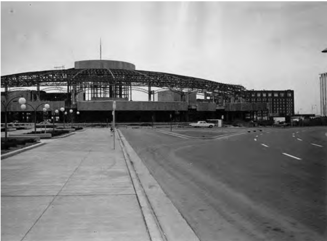
Figure 21 – Photo of Auditorium Complex Civic Cultural Center Construction Site, Circa 1968 – Photographer Unknown, WICHITA PHOTO ARCHIVE, wichitaphotos.org, Archives of the Wichita Chamber of Commerce, Wichita State University Library, Special Collections, Date Digital 2003
