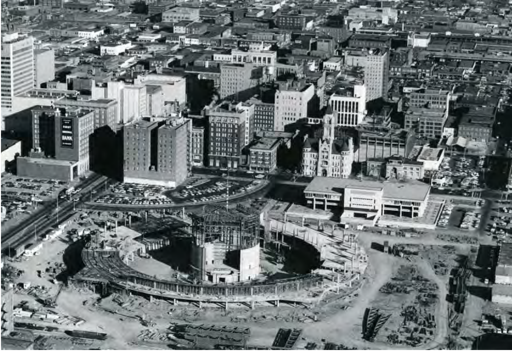
Figure 20 – Aerial Photo of Auditorium Complex Civic Cultural Center Construction Site, 1966 – Photographer Unknown, WICHITA PHOTO ARCHIVE, wichitaphotos.org, Archives of the Wichita Chamber of Commerce, Wichita State University Library, Special Collections, Date Digital 2003
