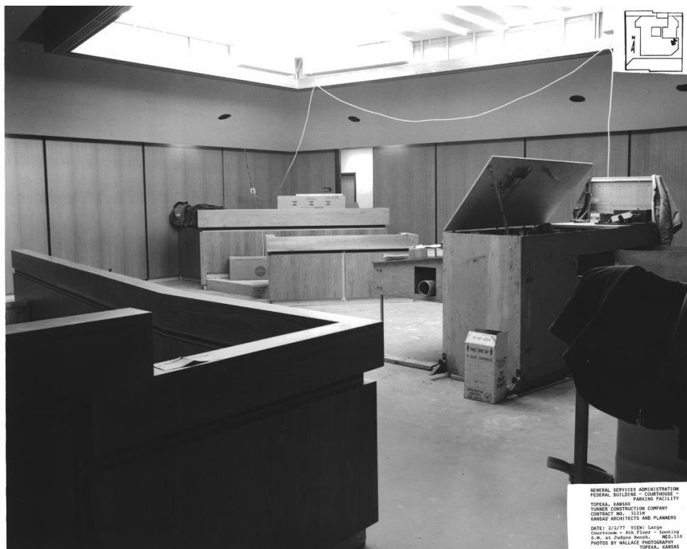
Figure 23. Courtroom under construction, February 2, 1977, Wallace Photography, [On file at Frank Carlson Federal Building and US Courthouse]
