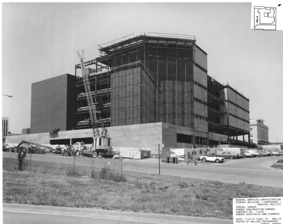
Figure 19. View toward northeast corner showing progress of brick veneer installation, July 14, 1976, Wallace Photography [On file at Frank Carlson Federal Building and US Courthouse]
