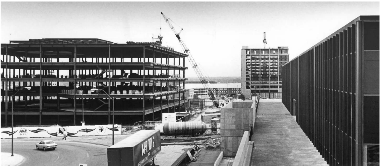
Figure 31. View of Frank Carlson Federal Building and US Courthouse under construction, ca. early 1976. Townsite Plaza Office Park is to the right. [Topeka Capital Journal]
