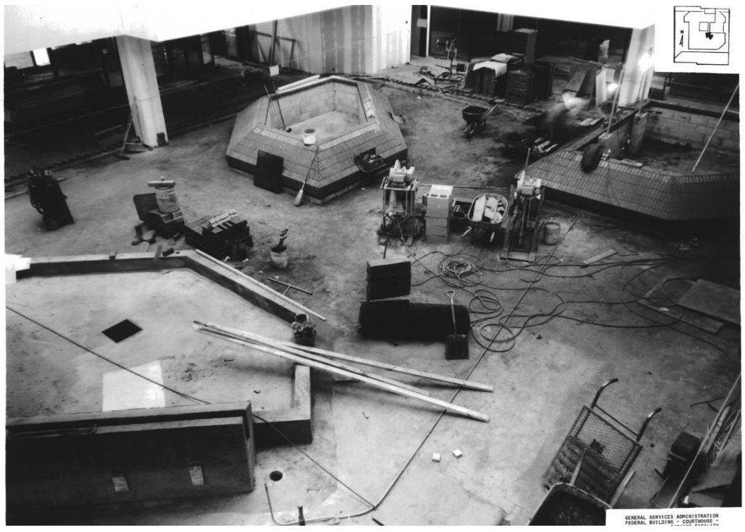
Figure 24. Atrium under construction, view likely from second floor, circa late 1976, Wallace Photography [On file at Frank Carlson Federal Building and US Courthouse]
