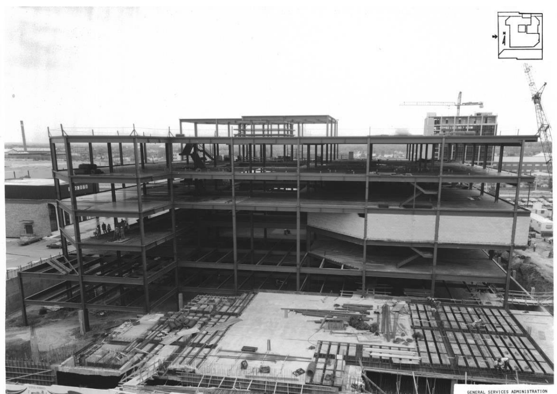
Figure 17. View of steel frame, front façade, circa March 1976, Wallace Photography [On file at Frank Carlson Federal Building and US Courthouse]
