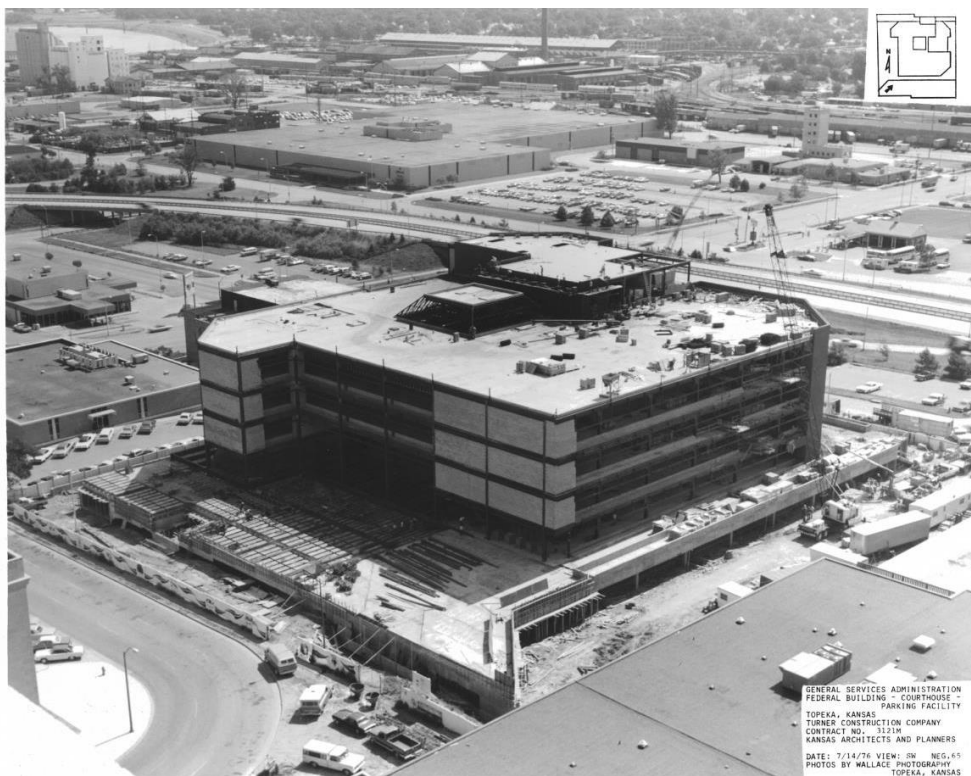
Figure 18. Aerial view, looking northeast, showing installation of concrete-block walls, June 15, 1976, Wallace Photography [On file at Frank Carlson Federal Building and US Courthouse]
