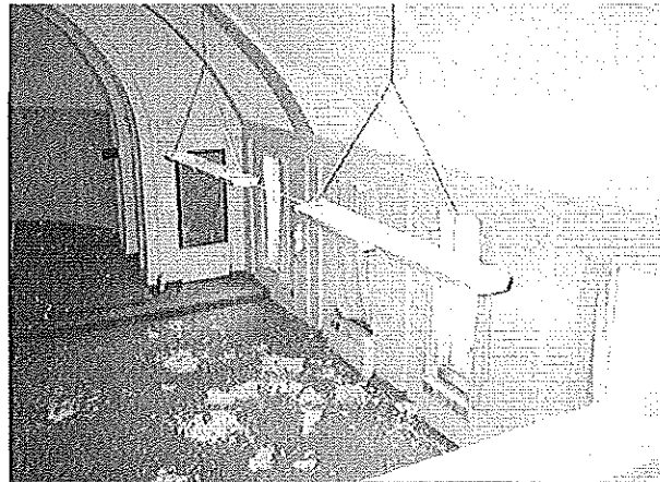
Chapel ceiling paint
